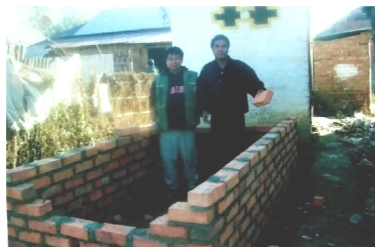
Construction of garbage tank with half brick masonry at Khomidok Bazar under Imphal East ZP
