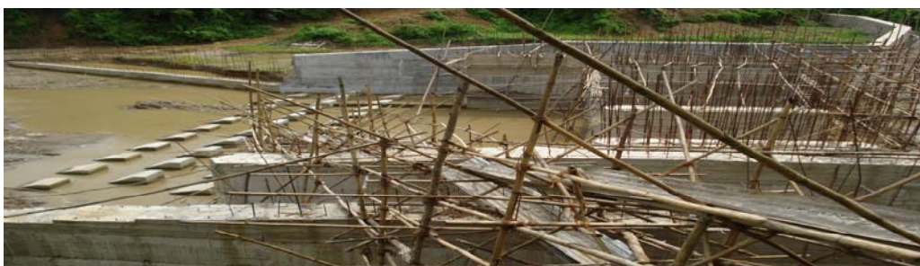
Photograph showing the present status of the Langlong MI project Ph II (July 2008)
