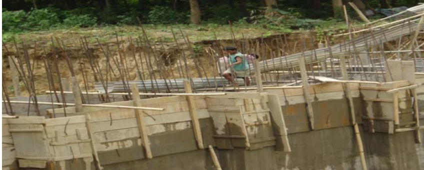
Photograph showing the present status of the Awokupughoki MI project Ph II (July 2008)
